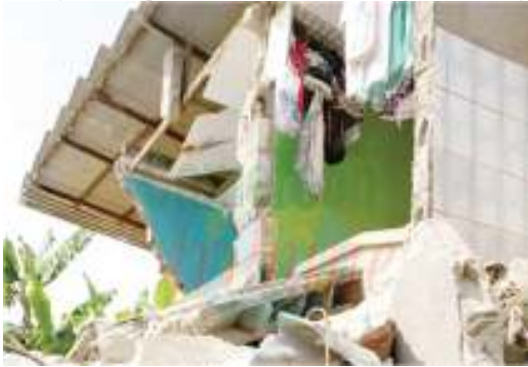
Fig. 1 Collapse of four- storeys building in the Ndogbat suburb
