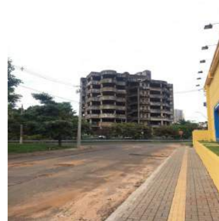
Figure 2 – Abandoned building in study. Source: Personal Archive (2019).
